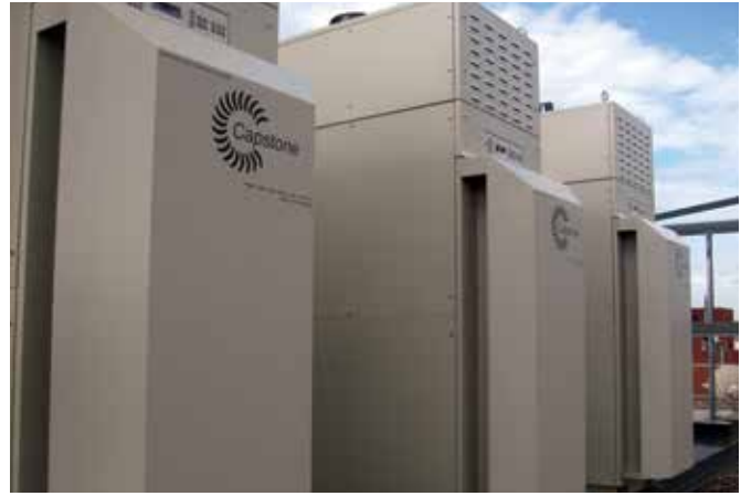
Commissioned in 2019, the rooftop-mounted C65 ICHP microturbines have logged more than 85,000 runtime hours, which amount to 99.8% uptime.
