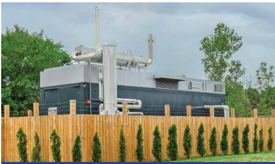
The City of Windsor in Ontario, Canada, recently installed a combined heating and power system at its Huron Lodge care facility, a 177,000-square-foot, long-term care home for all ages that is one of the largest consumers of gas and electricity in the municipality.
