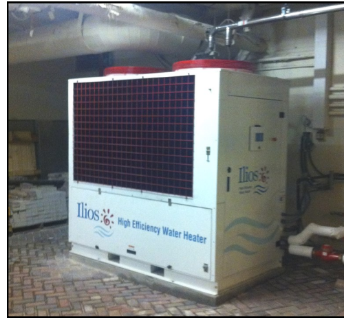
The Harbour House Ilios HEWH-500-AS will save residents/owners more than $25,000 each year.
