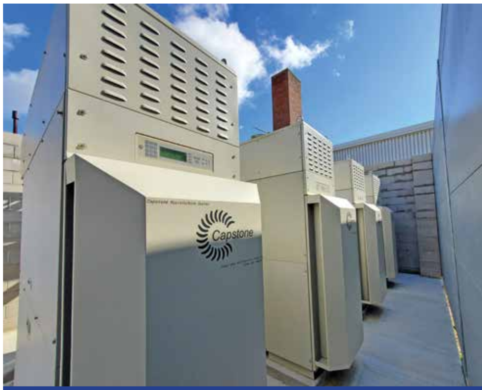
Dryden Regional Healthcare Centre turned to CHP to reduce its rapidly increasing electricity costs. Four natural gas-fueled Capstone C65 microturbines provide electricity and supply the building’s heat, leading to cost savings of at least $150,000 per year.
