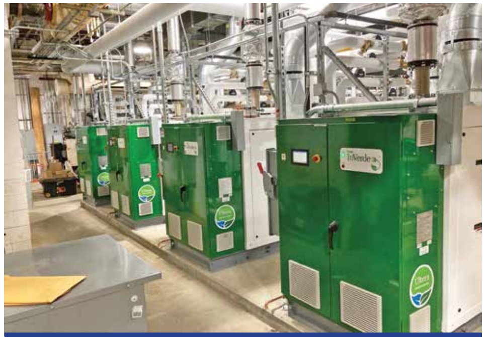
PHOTO COURTESY OF TECOGEN INC.
