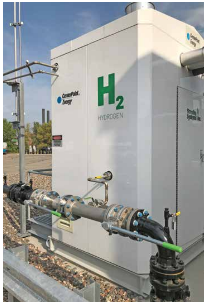
PHOTO COURTESY OF CENTERPOINT ENERGY INC.
